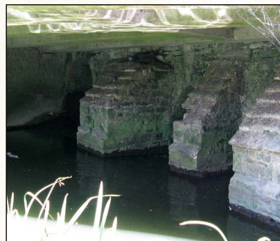
Above: The 14th Century stone Mill Street bridge over the River Len, now hidden beneath a modern road bridge
